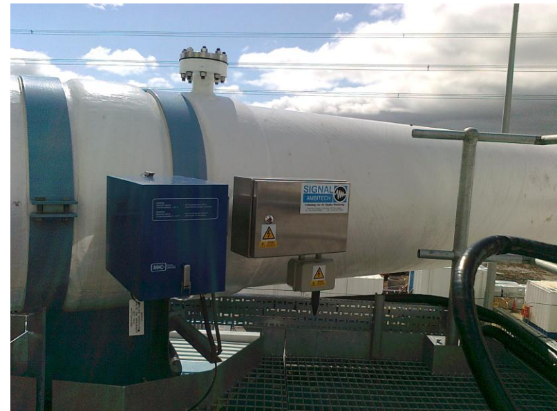
Installation at CCS pilot plant
